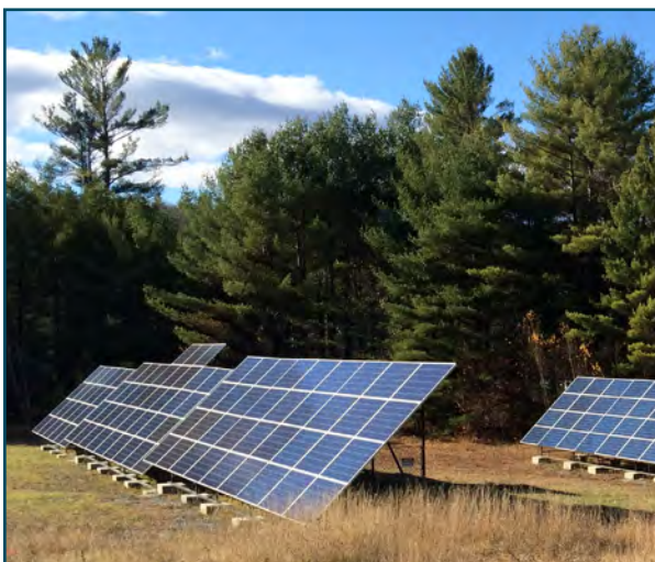
Solar panels in the hamlet of Chestertown.
