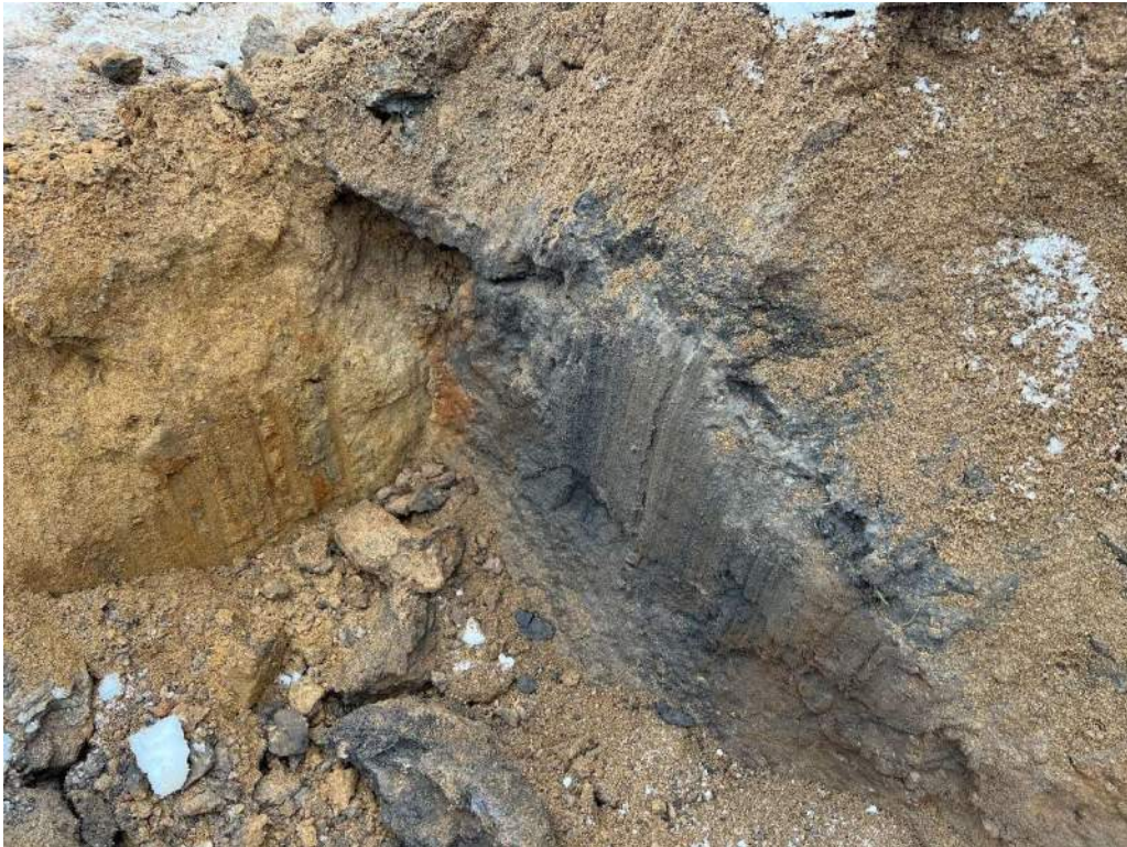
Tank B Stained Soil
