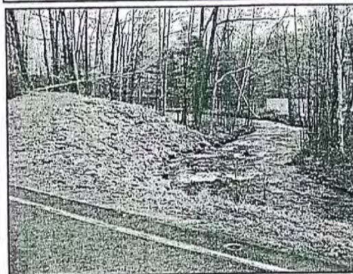
The completed stream bank repair and stabilization project at 'Station 94' of Hague Brook, located at the Town Center and West Hague Road.
