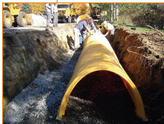
Stormtech chambers being installed along West Brook in the Town of Lake George by Warren County Soil and Water Conservation District.
