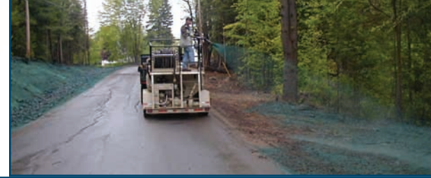
Warren County Soil & Water Conservation District deploys Hydroseeding Unit procured with EPF funds.
