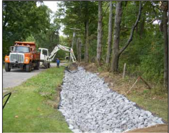
Highway department lining roadside ditch with stone, Essex County. Photo courtesy of Essex County SWCD.
