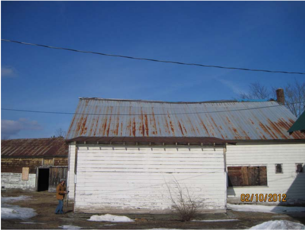
Photograph 13 – Scales Building – South Side, Note Dip in Ridge
