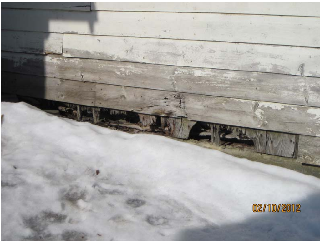
Photograph 20 – Scales Bldg. – Decayed Wall Plate and Post Base
