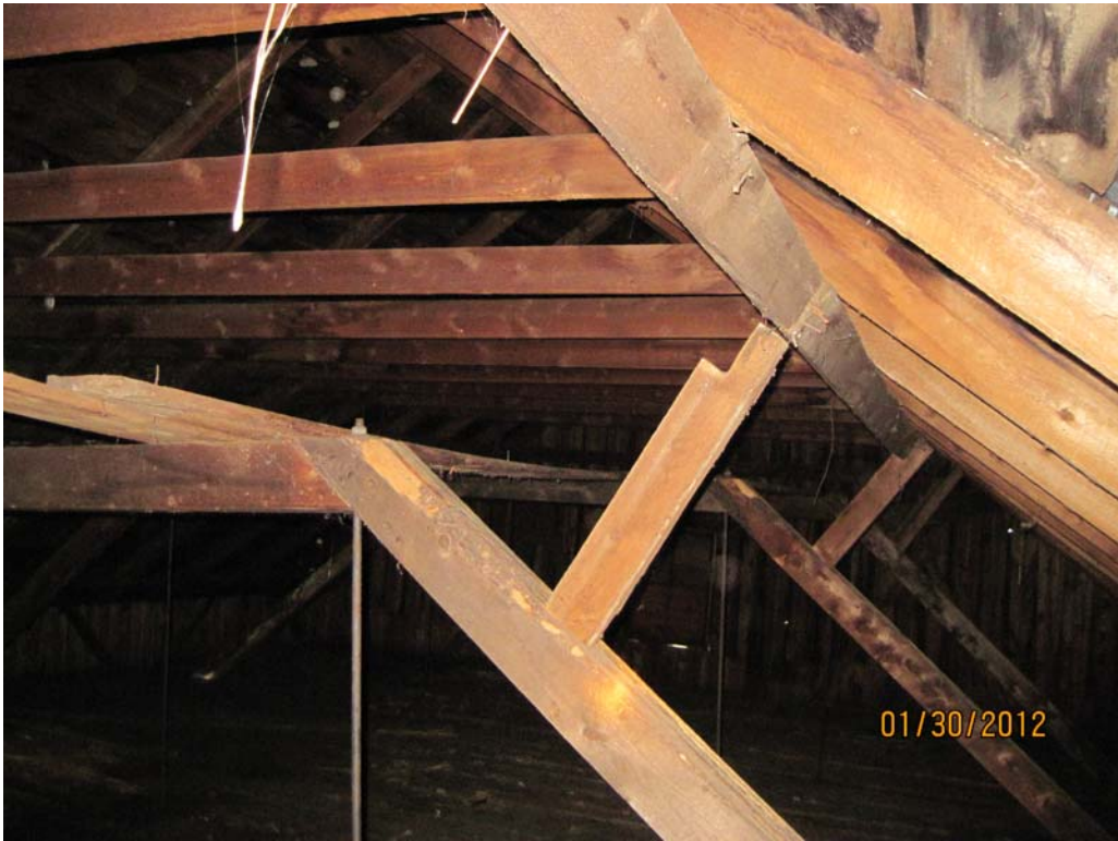
Photograph 16 – Scales Bldg. - Purlin Support of Rafter Pulled Away From Truss
