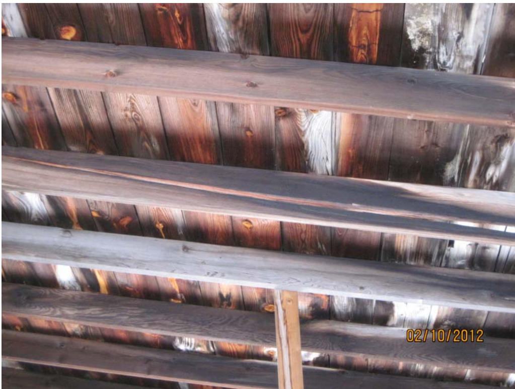
Photograph 24 – Scales Bldg. – Scale Pit Enclosure w/ Split Rafter and Decayed Planks
