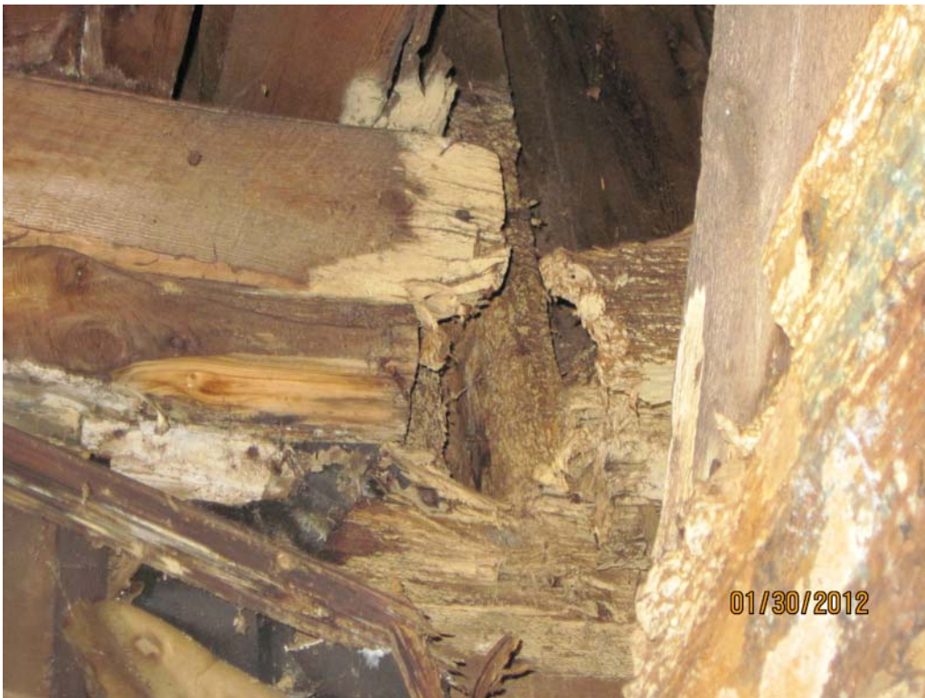
Photograph 18 – Scales Bldg. – Rotten Truss to Column Connection
