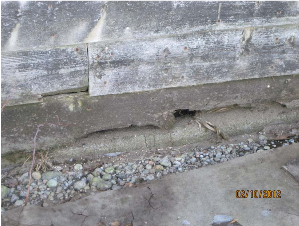
Photograph 19 – Scales Bldg. – Decayed Siding and Bottom Wall Plate
