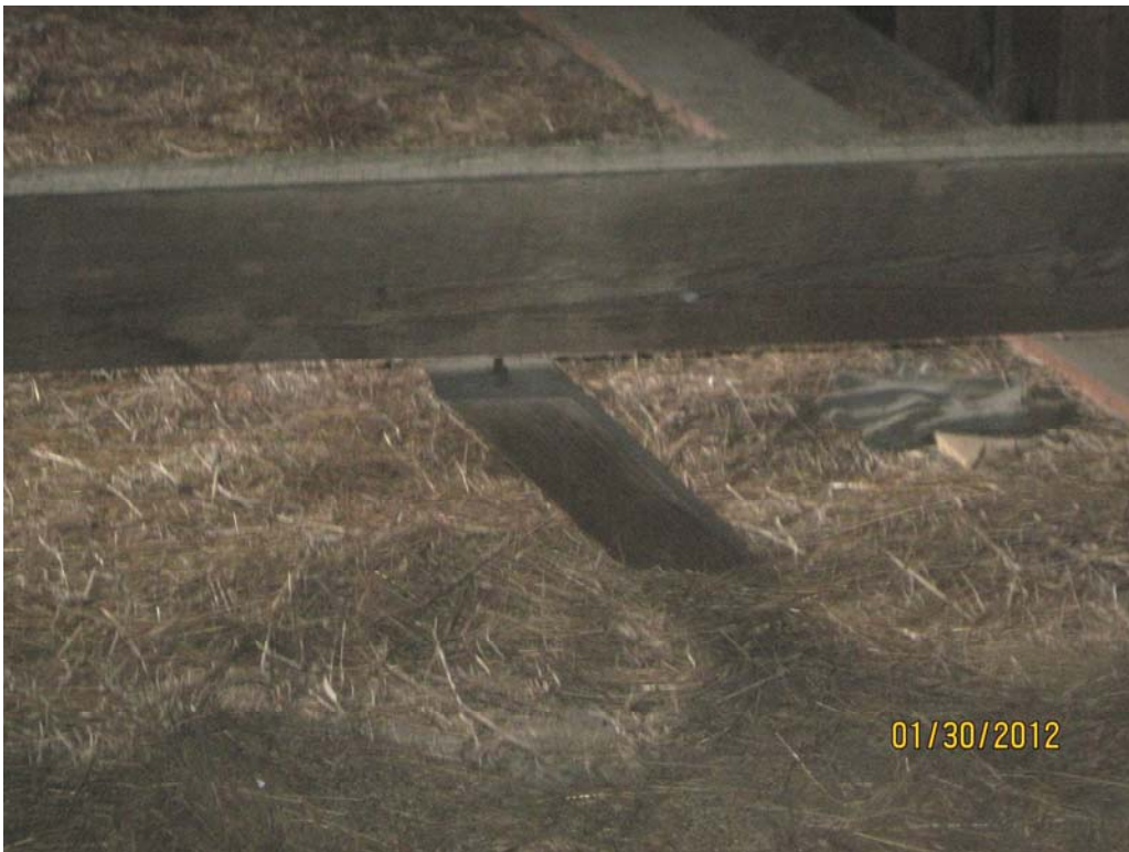
Photograph 10 – Stables Knee Brace Has Pulled Away From Tie Beam
