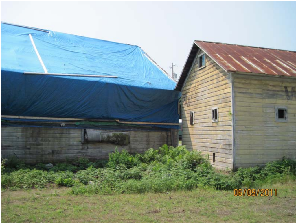
Photograph 12 – Scales Building North Side with Roof Collapse, Note Sag in Siding on Left Side of Picture.
