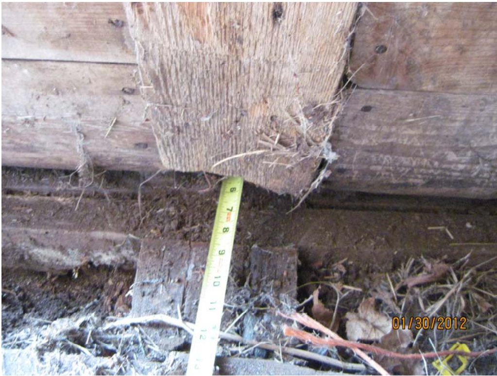
Photograph 11 – Stables Decayed Post Base
