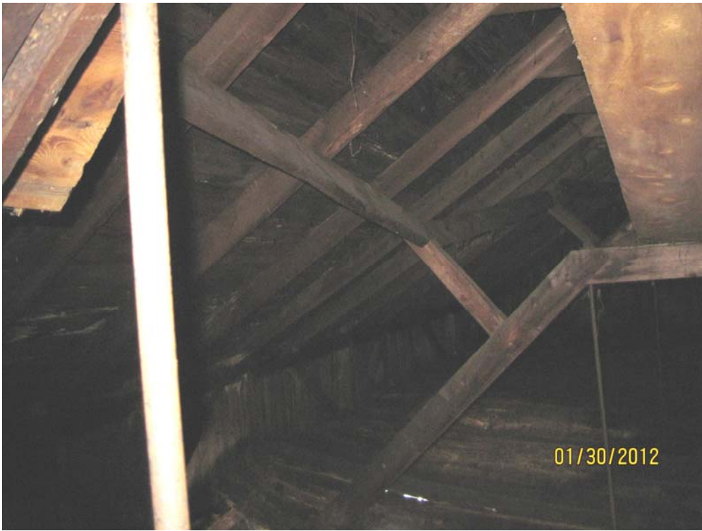
Photograph 17 – Scales Bldg. – Failed Bearing End of Truss
