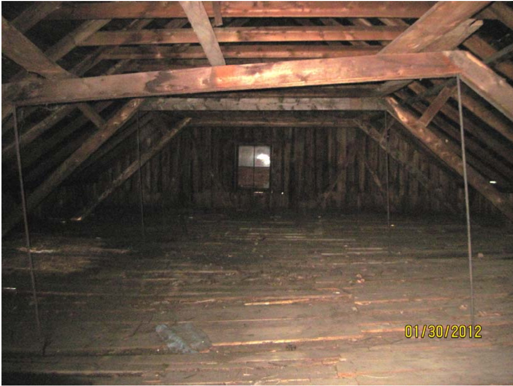
Photograph 15 – Scales Bldg. Truss Framing, Failed Truss on Left
