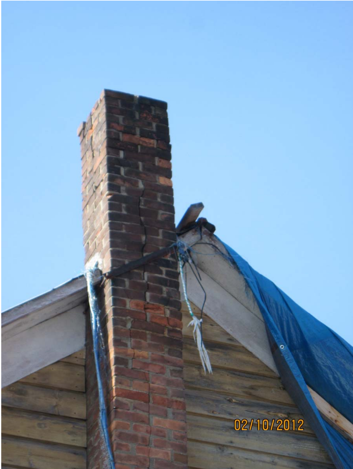
Photograph 25 – Scales Bldg. – Cracks in Brick Masonry Chimney
