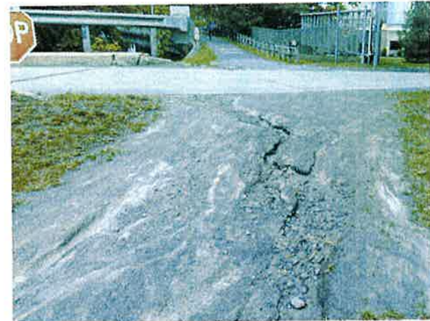
Trail erosion at the Lehigh Cement Plant driveway crossing
