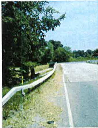
Narrow Shoulder with debris
