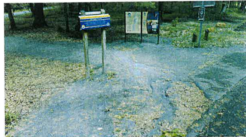
Trail Erosion at Bush Street Crossing
