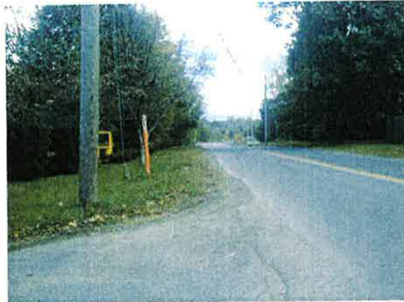
Missing sidewalk along Murray St. (Looking east towards trailhead)
