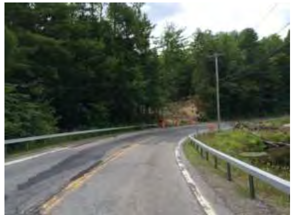
At washout near Big Brook View southwest
