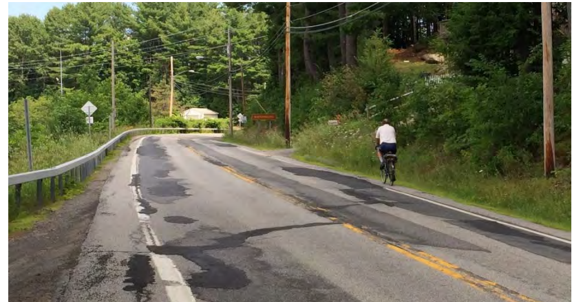
Narrow and poor road shoulder conditions along River Street can deter cycling and can contribute to a number of safety related concerns
