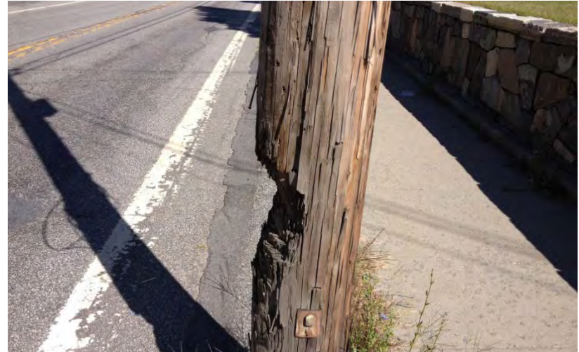
Evidence of vehicle and/or snow plow impacts can be seen on several utility poles within the corridor. Other utility poles are considerably closer to the travel lane.
