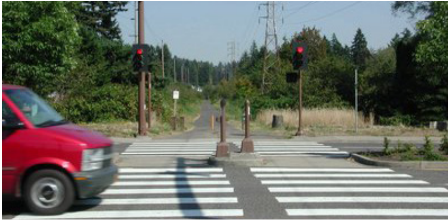
Full traffic signals include signals facing trail users to indicate when it is or is not safe for path users to cross the roadway.
