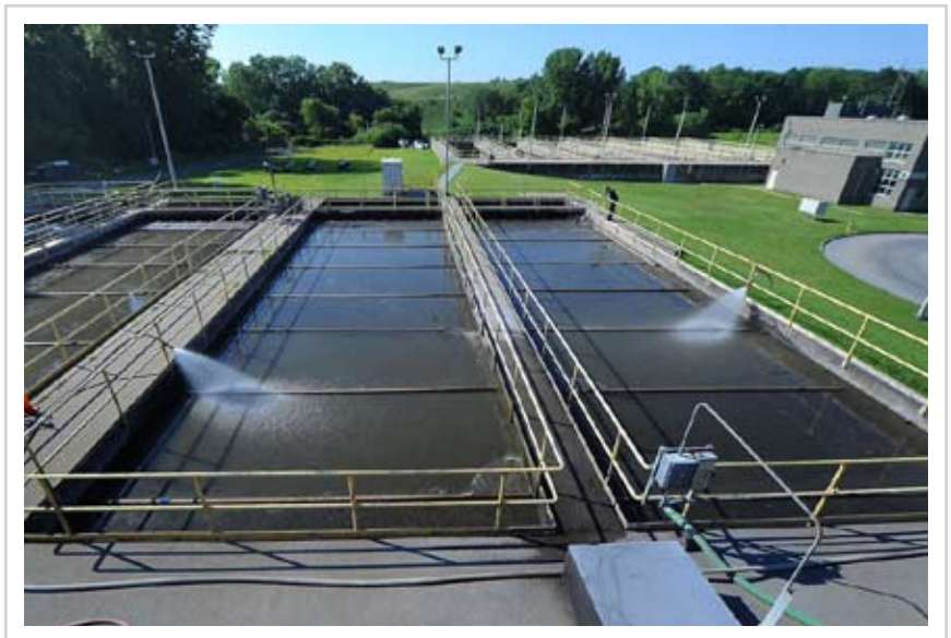
Primary tanks at a waste water treatment plant. Photo: Post Star
