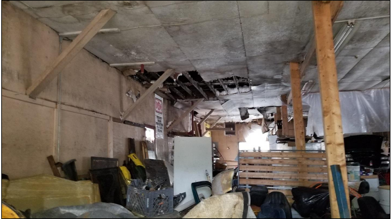
Photo 29. Piles of debris in main garage area. Looking toward Riverside Drive.
