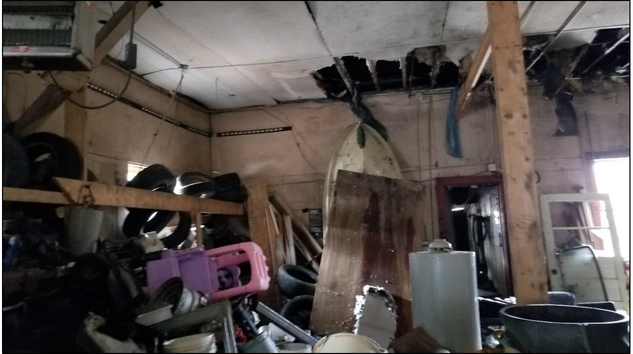
Photo 23. Piles of debris in main garage area.
