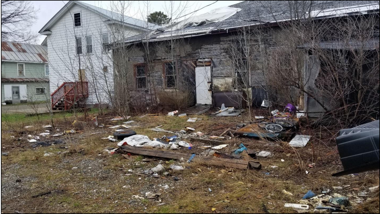
Photo 9. Rear of property, facing structure – note debris.
