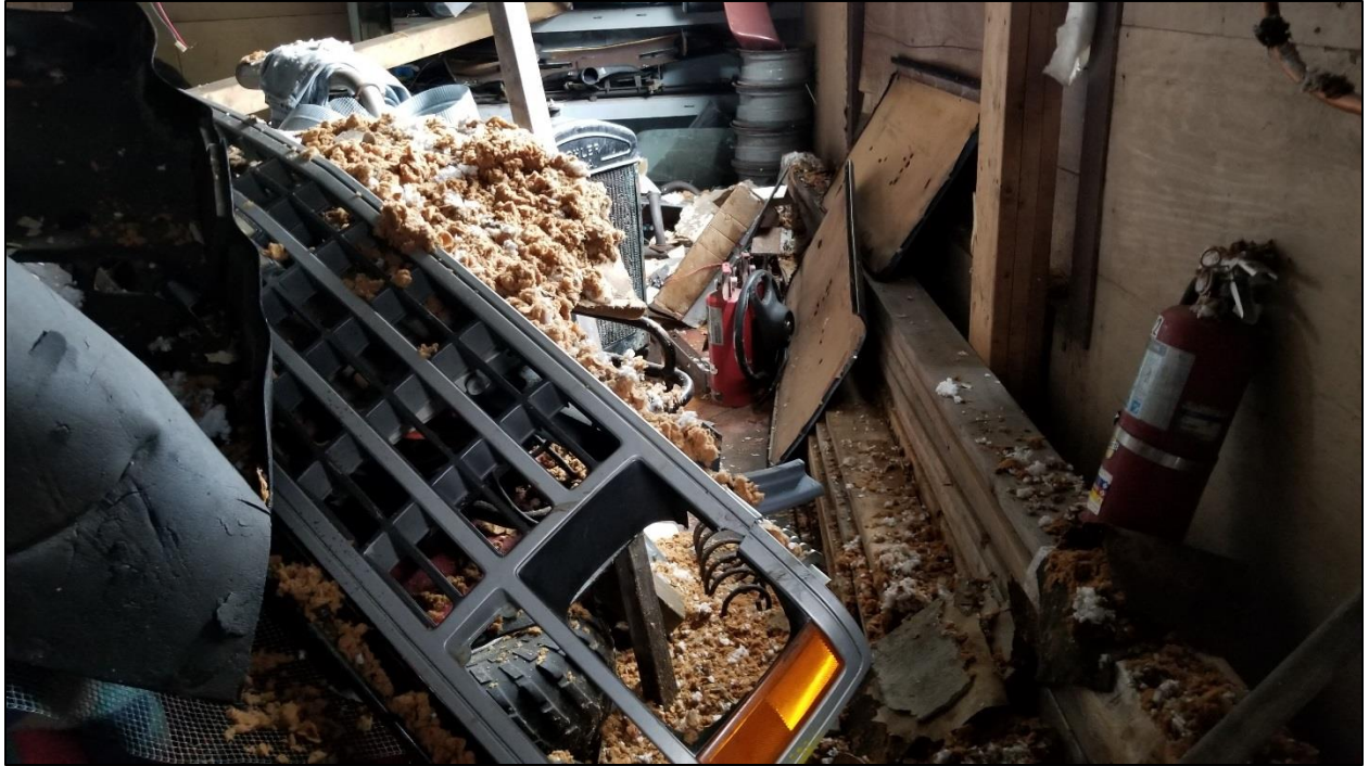
Photo 17. Main garage area; fallen insulation from roof.
