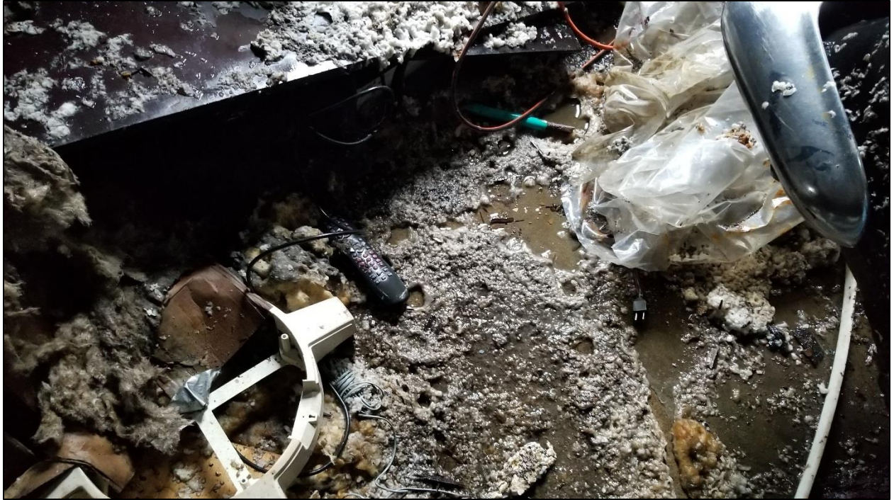
Photo 25. Insulation and water from leaking roof in main garage area.
