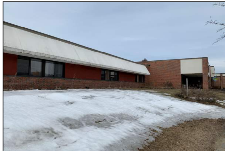
Photograph No. 4: Southeast side of the building with stained insulated plaster veneer overhangs.
