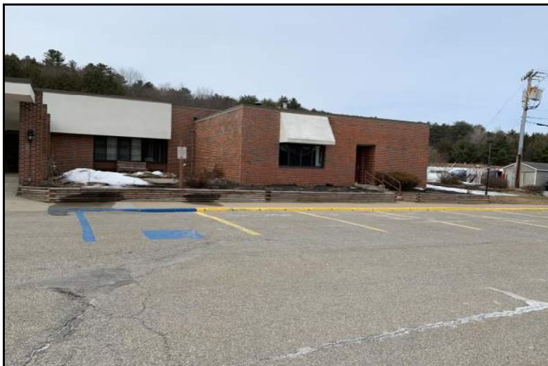
Photograph No. 3: Northeast corner of the building with handicap parking space (currently not meeting ADA signage standards).
