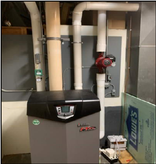
Photograph No. 33: Hot water boiler.
