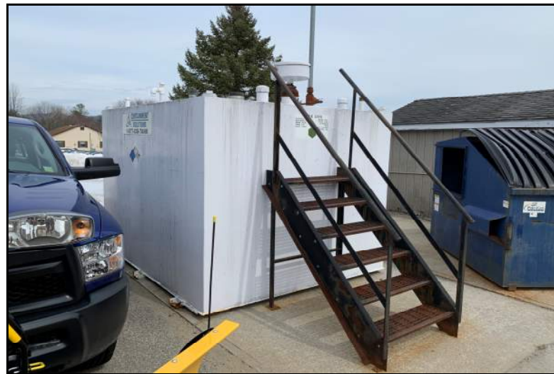
Photograph No. 40: Existing 3,000-gallon above ground fuel oil storage tank.
