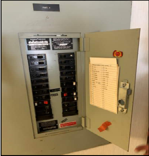
Photograph No. 36: Typical Corridor subpanel.
