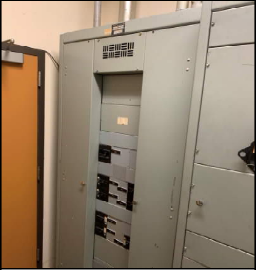
Photograph No. 34: Main electric service switch gear.
