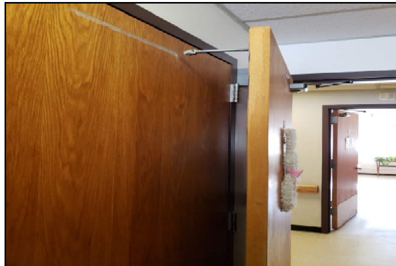
Photograph No. 22: Typical Resident Room entry door with hold open.
