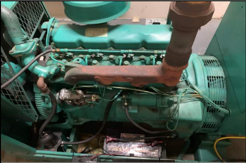
Photograph No. 35: Existing emergency generator.
