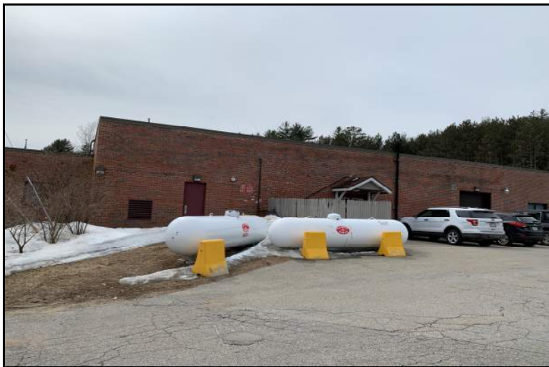
Photograph No. 39 Existing propane storage tank.
