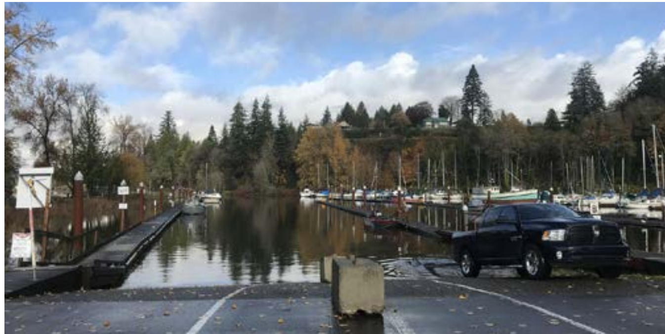
The three lane concrete boat ramp separated into two lanes. Credit: Jordan Sector
