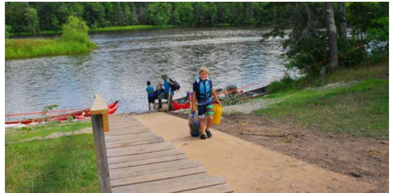
Recent construction of access improvements to the St. Croix Wild and Scenic River. Credit: Thomas O'Keefe.
