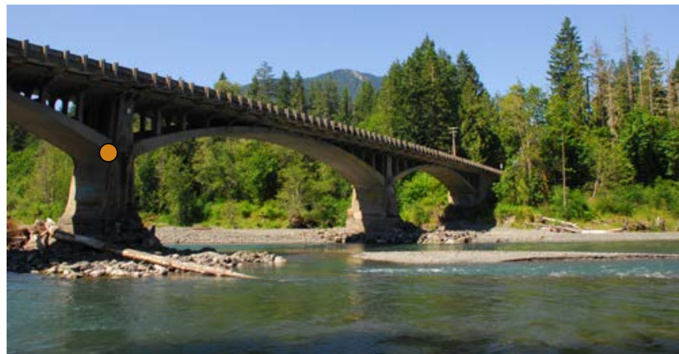
The historic McDonald Bridge was constructed in 1926, but since removal of Elwha Dam was completed in 2012, the elevation of the river bed at the bridge site has lowered 14 feet. Since the bridge foundations are set on gravel, concern over the integrity of the bridge has prompted the Washington Department of Transportation to initiate an emergency project to rebuild the bridge. Credit: Thomas O’Keefe.
