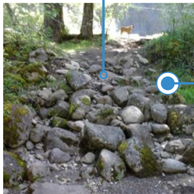
Prior to the project, access was located down a steep slope over existing boulders to a gravel beach at the edge of the river. It was difficult to maneuver large rafts and kayaks over the uneven surfaces. Credit: Jordan Sector.
