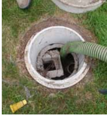
FIGURE 4-12 – Photo of maintenance/pumpout of septic tank.
