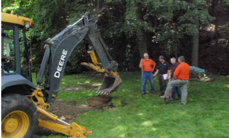
FIGURE 4-5 – Town of Lake George Director of Planning Keith Osborne, Town employees, and Eric Murdock of On Site Systems performing site inspection.
