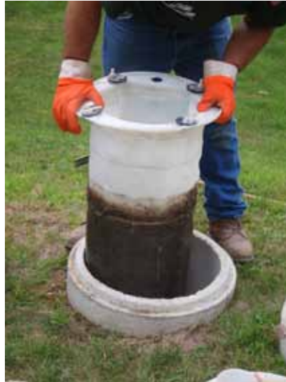
FIGURE 4-13 – Photo of inspection and maintenance of effluent filter.
