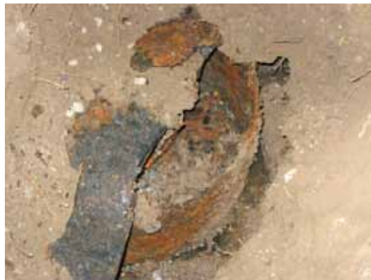
FIGURE 4-10 – Figure 4-10 – Photo of metal septic tank with evidence of corrosion. (Photo provided by Wim McIntyre)
