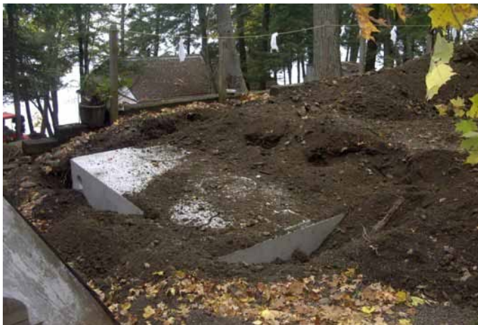
FIGURE 4-9 – Photo of newly installed concrete septic tank (Photo provided by Wim McIntyre)
