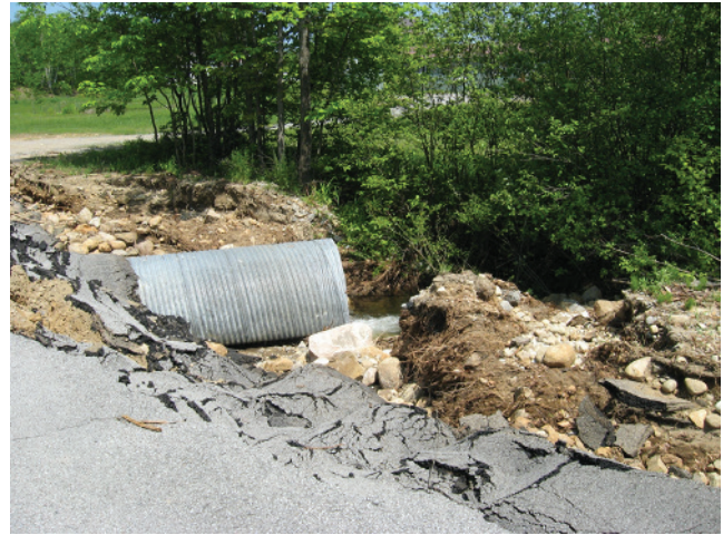
Photo 8: Heavy rain events and runoff can lead to severe roadside erosion. Photo Courtesy of Warren County SWCD.
