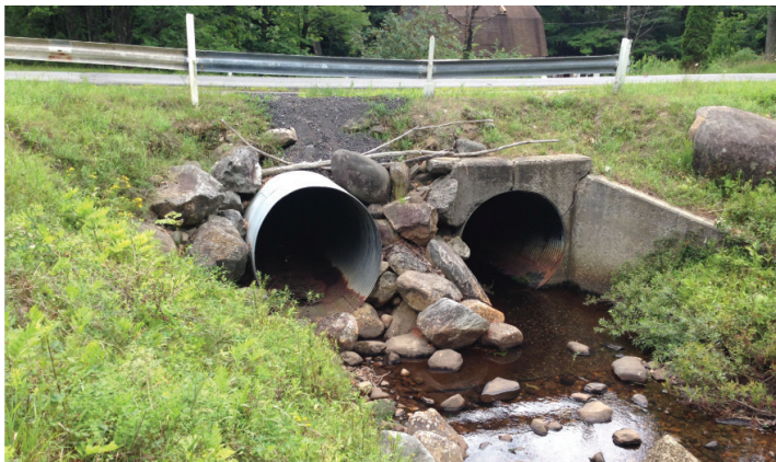
Photo 19: Undersized culverts on Mayfield Creek, Town of Mayfield, Fulton County.
