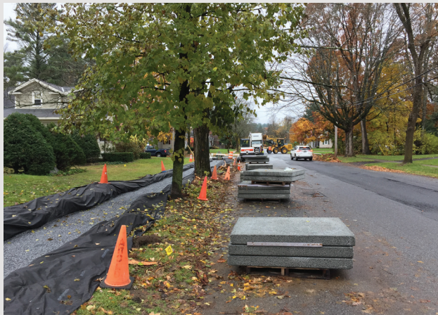
Photo 3: Porous sidewalk project under construction, City of Glens Falls. Photo courtesy of Nick Rowell.
