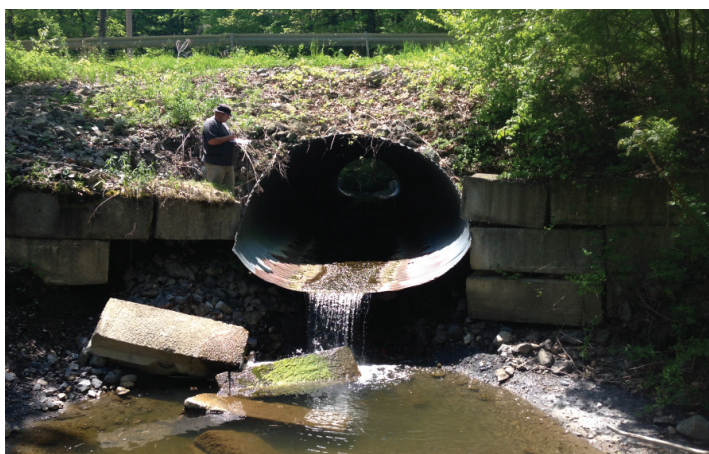
Photo 18: Perched culvert on MacDonald's Creek, Saratoga County. Perched culverts do not allow fish migration/passage through a stream. Photo Courtesy of Saratoga County SWCD.
