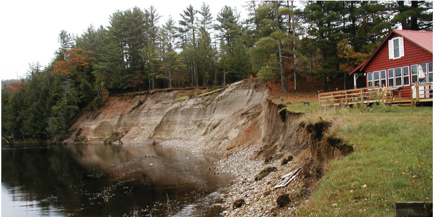
Photo 7: Streambank erosion at Cave Banks on the Sacandaga River in Hamilton County – Project Recommendation E-08. Photo courtesy of Hamilton County SWCD.
