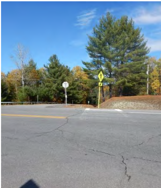
Figure 5 - Faded crosswalk marking at Intersection A
