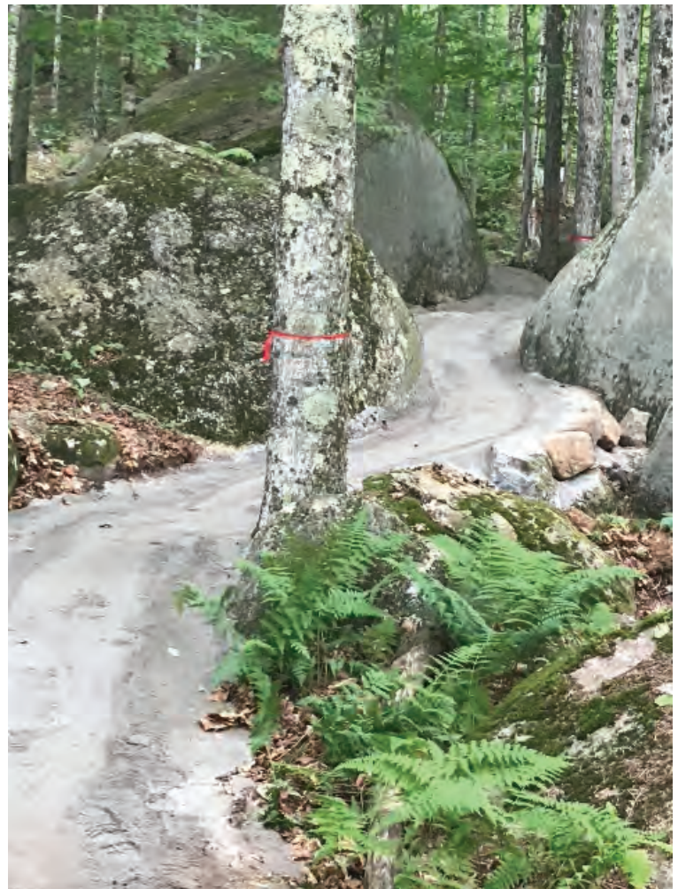
Above: Installation of an stone dust surfaced shared use trail through an erratic boulder field at Fern Park, Inlet, NY.
