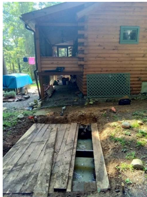
Cesspool for wastewater treatment found in the Town of Hage. Such systems are not allowed by NYS health code
