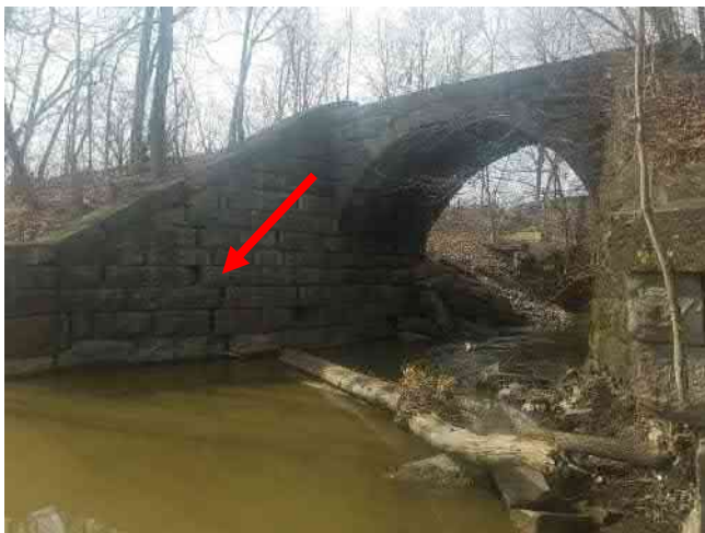
Photograph (3): General view. East Elevation. Displaced stones.
