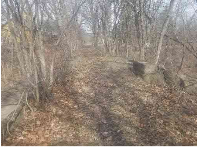
Photograph (9): View of trail along top of bridge. Vegetation / trees growing along bridge.
