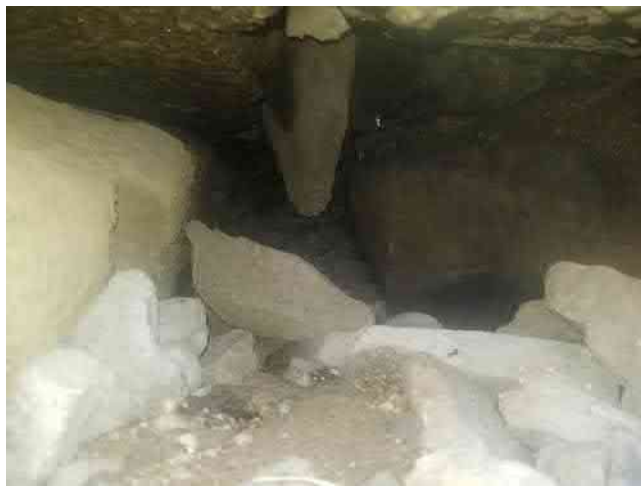
Photograph (5): Closeup view of void at southwest abutment as shown in Photograph #4.
