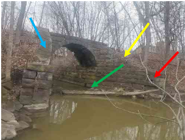
Photograph (2): General view. East Elevation (inlet). Debris restricting flow. Displaced stones (red arrow). Leaning / bulging wing wall (blue arrow). Missing cap stones (yellow arrow). Missing stone / undercut at north abutment (green arrow).
