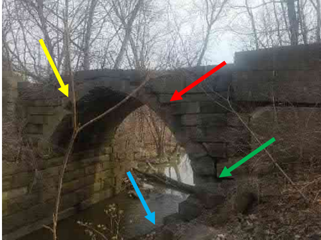
Photograph (1): General view. West Elevation (outlet). Displaced stone (red arrow), voids in abutment (green arrow) missing stone (yellow arrow).
