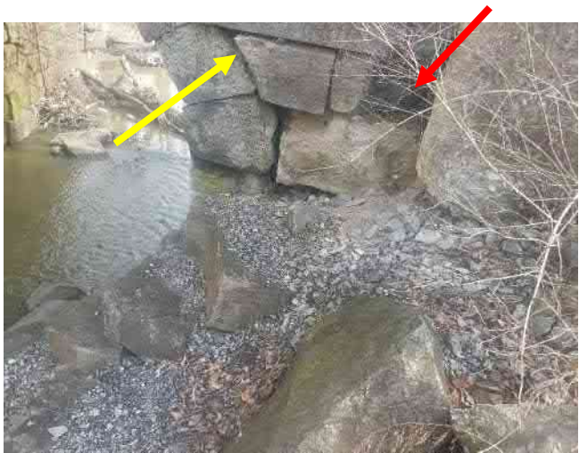
Photograph (4): Void within southwest abutment (red arrow), displaced stones (yellow arrow).
