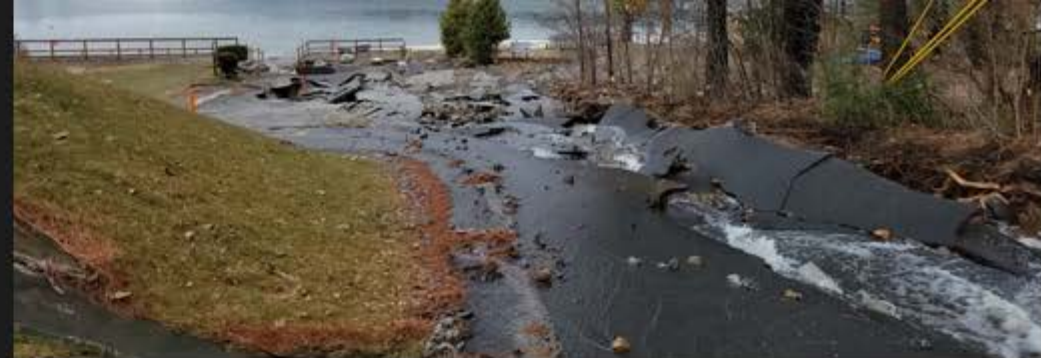
Severe damage to the driveway and parking lot of the Lakeview Terrace Hotel and the Fairview Association, along Lake George, N.Y. (Photo: Jay Petrequin)
