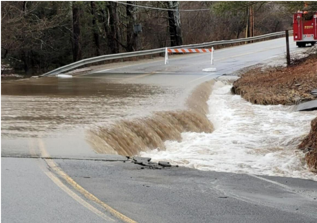
Figure 5.4.6-4 Washout of Olmstead Road due to Beaver Dam Failure, March 2022
