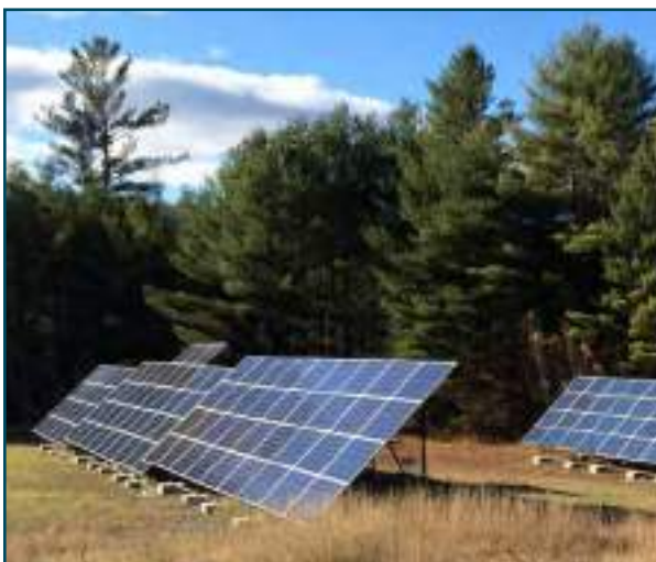
Solar panels in the hamlet of Chestertown.
