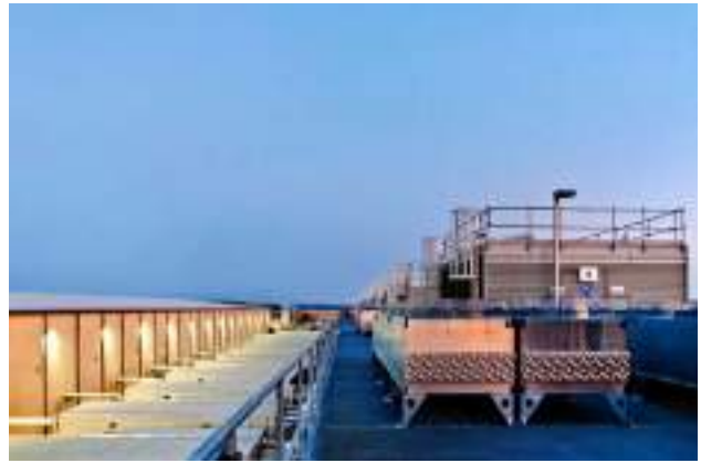
Cooling towers at the Data Center
