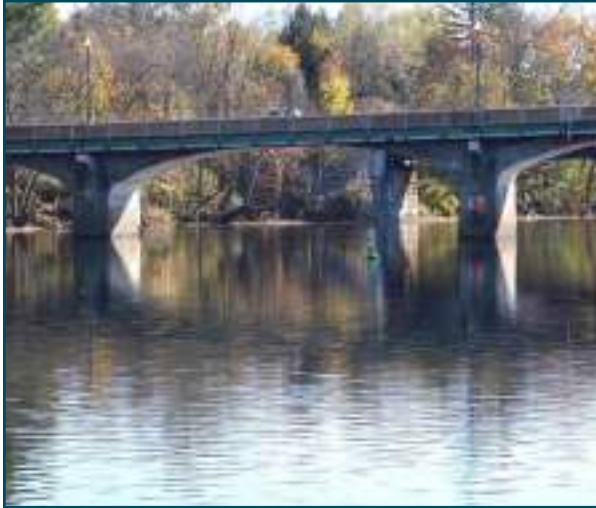
103 bridges in the Region are "structurally deficient."
