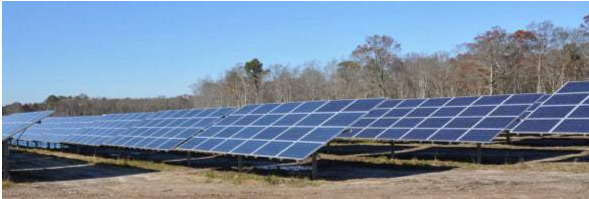
Solar Panels at Long Island Solar Farm
