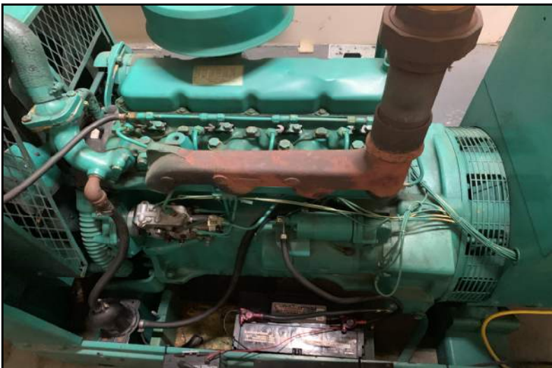
Photograph No. 35: Existing emergency generator.
