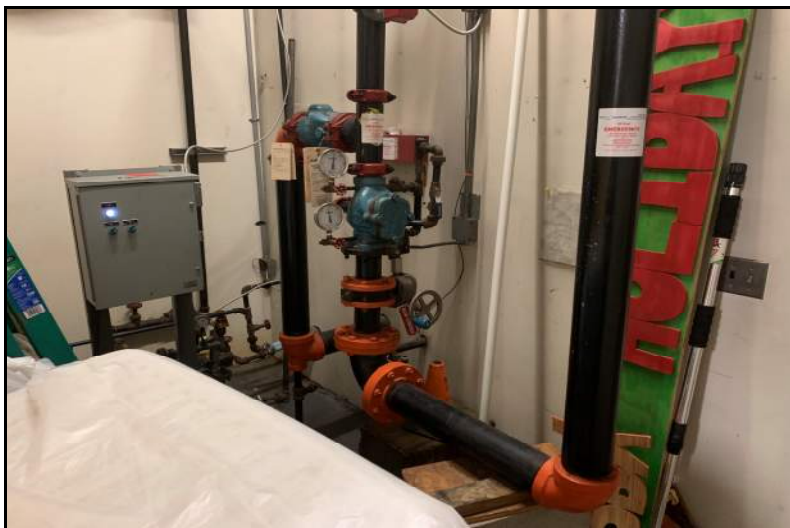
Photograph No. 31: Fire protection riser.
