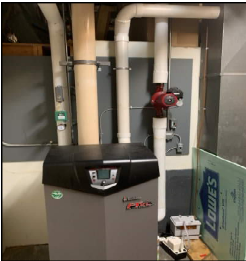
Photograph No. 33: Hot water boiler.
