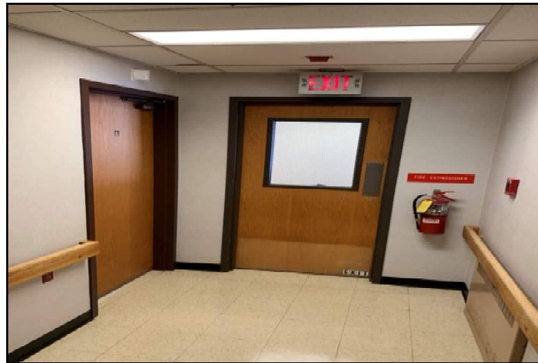
Photograph No. 38: Fire alarm notification device and pull station at corridor exit.
