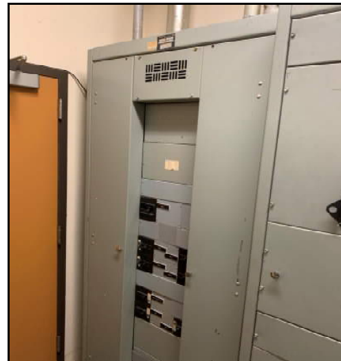
Photograph No. 34: Main electric service switch gear.
