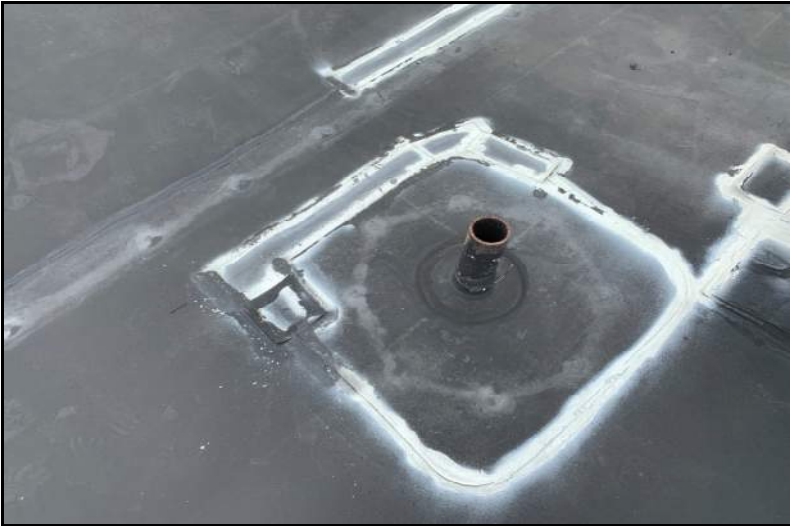
Photograph No. 12: Typical patches at existing roofing.
