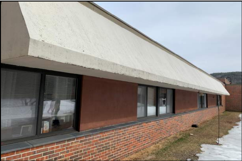
Photograph No. 5: Typical exterior perimeter wall with brick and mortar veneer and insulated plaster veneer.
