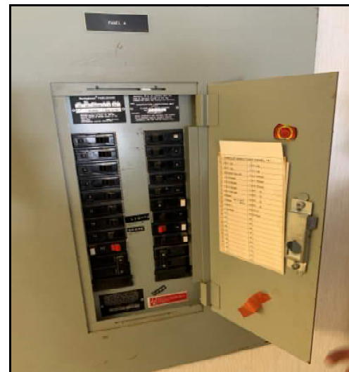
Photograph No. 36: Typical Corridor subpanel.
