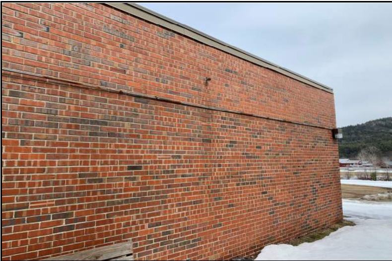
Photograph No. 6: Brick and mortar veneer with staining at south side of the building.
