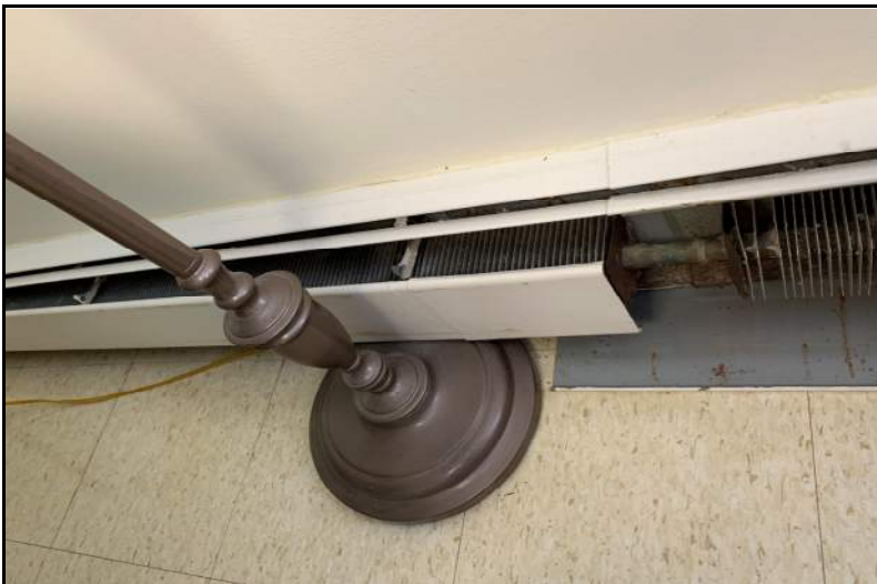
Photograph No. 21: Fin tube baseboard with damaged enclosure at Resident Room.
