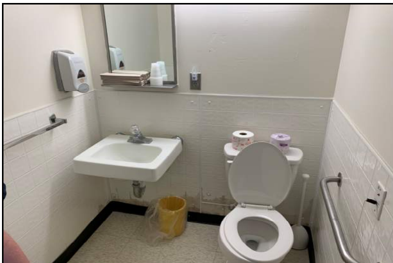
Photograph No. 19: Damaged FRP wainscot at Resident Bathroom.
