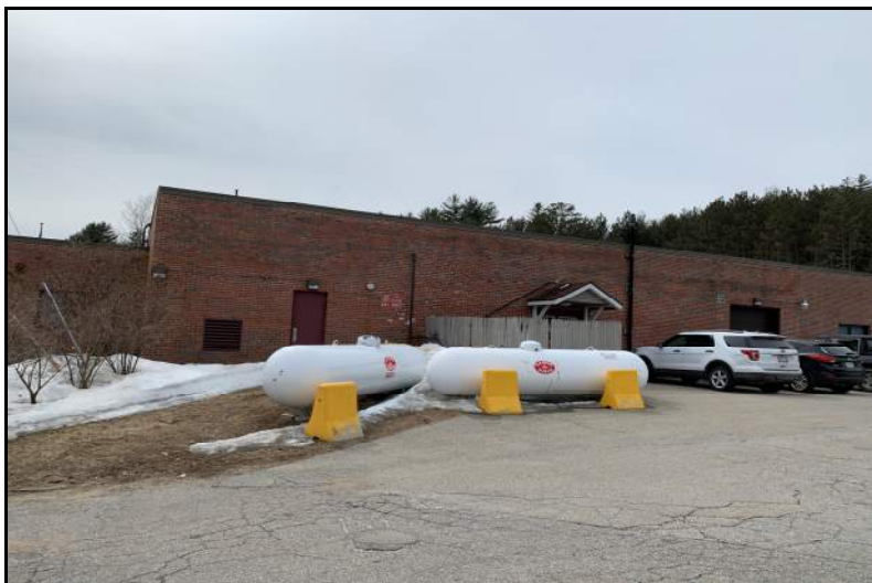
Photograph No. 39 Existing propane storage tank.
