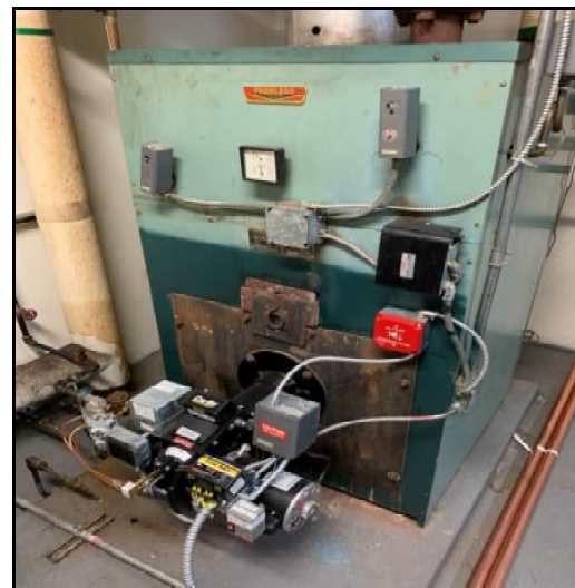
Photograph No. 32: Hot water boiler.
