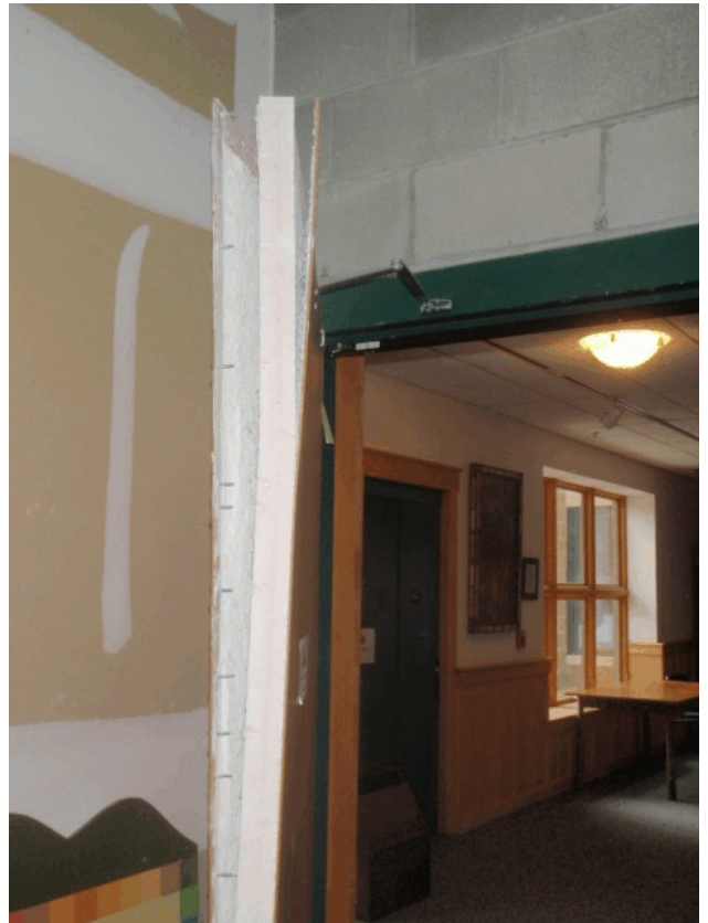
Lower level settling with moisture damage
