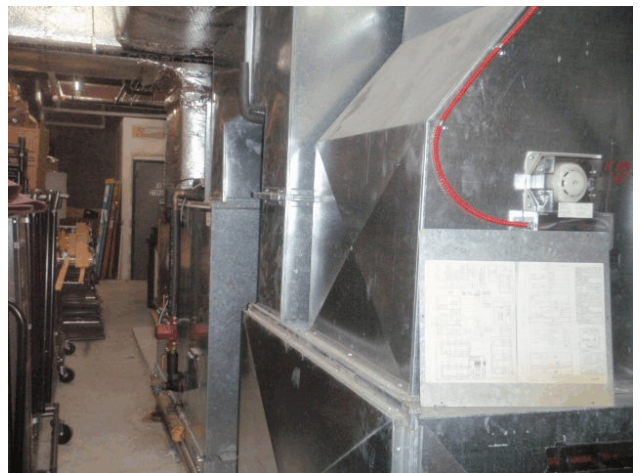
Heat pumps located in lower level with associated ductwork. 2 of the 3 pumps are inoperative.
