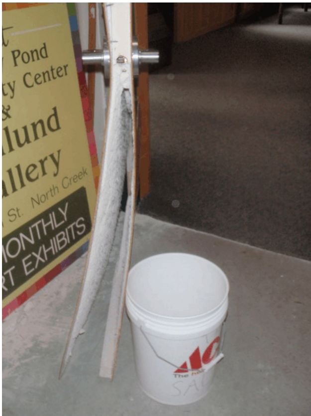
Moisture damaged fire door to be replaced
