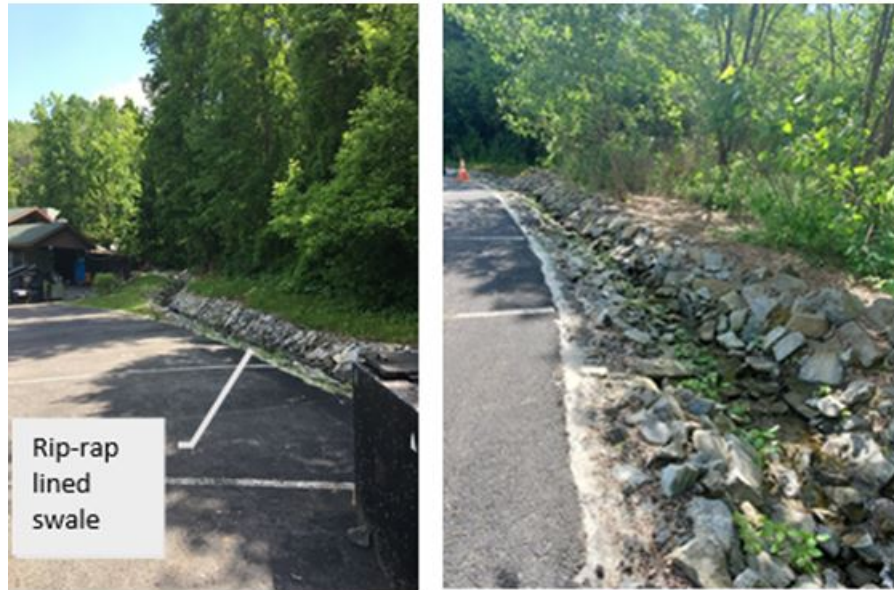
Figure 3. Existing stormwater conveyance system running around The Garrison property.
