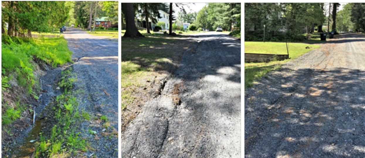
Figure 1. Erosion within the roadways along Cedar Lane and Beatty Road.
