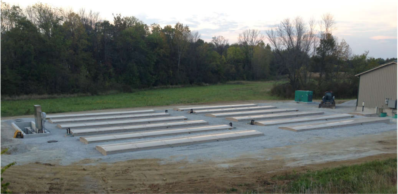
Figure 3. Typical AX-Max Treatment Facility (Christiansburg, OH)
