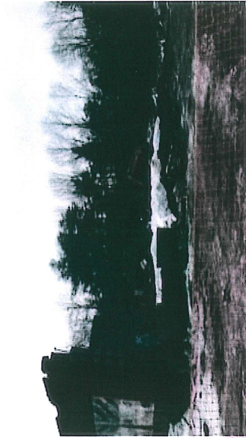
Photograph 1: View of existing work area from road side, with portion of front wall remaining.
