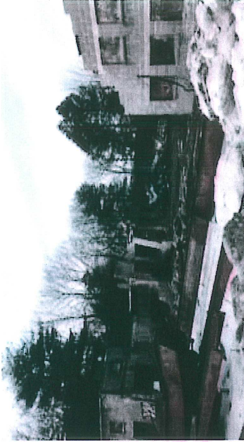
Photograph 2: View of remaining CMU walls and separated steel supports.
